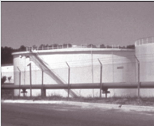
Chemical storage tank
